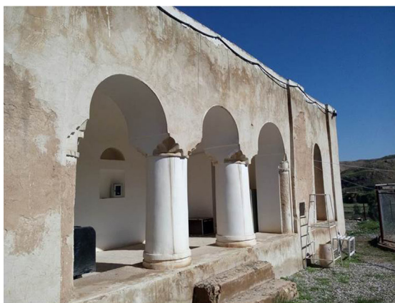
Plate 5. Right: A view of Jahangir Abad building, view from northeast; left: Entrance porch of southern side of the building (photo by Sharifinia).
